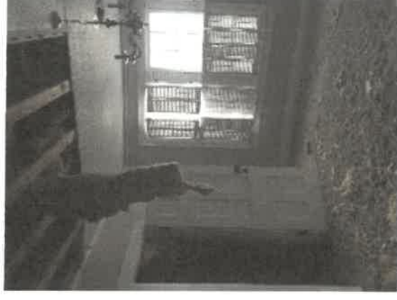
Hillcrest bedroom damage due to roofing beyond its useful life.
