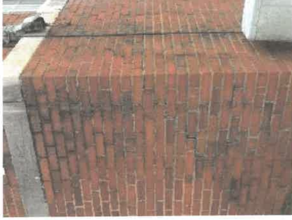
Bibb Graves deteriorated mortar and cracked bricks.
