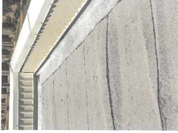
Engineering School roofing about to fail.
