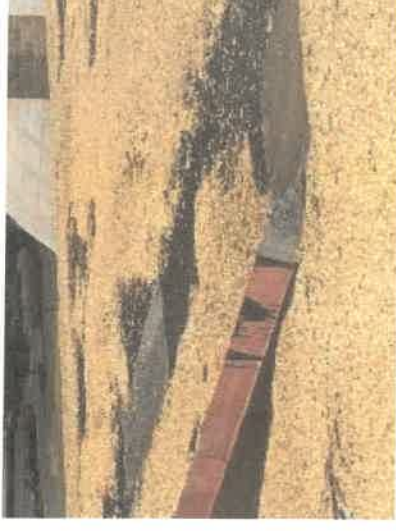
Council Training Center built up roof beyond useful life.
