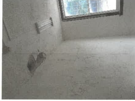
Bibb Graves stairwell damage due to poor gutters, leaders and mortar.
