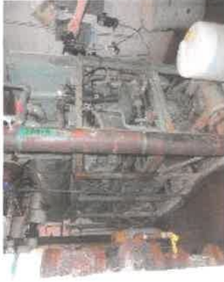
Carver Annex – 36 year old reciprocating chiller, well beyond 20 year life
