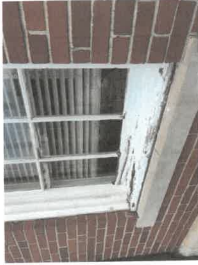
Carnegie failed rotted wood windows.
