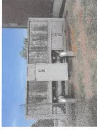
L. R. Patton Hall – 20 year old rotary screw chiller at the end of 20 year life
