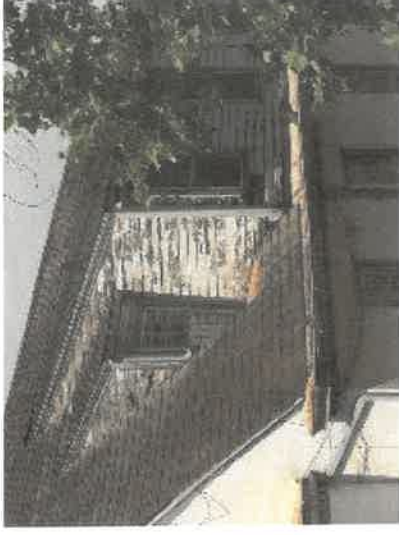
Hillcrest rotted siding.
