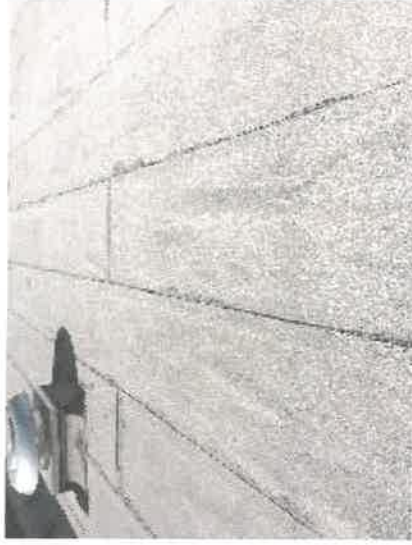
Carver Complex rolled asphalt roofing at end of useful life.
