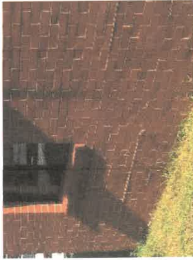
Poultry Science deteriorated mortar.
