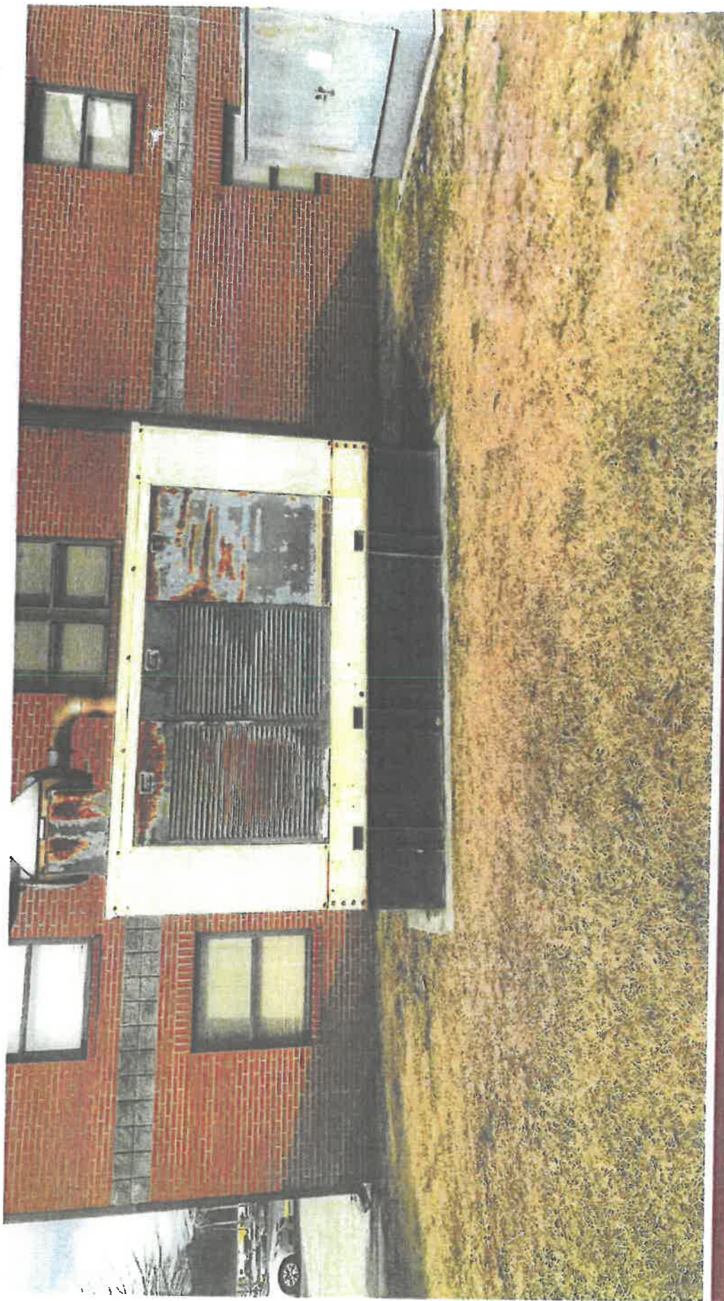
Diesel Back-Up Generators
