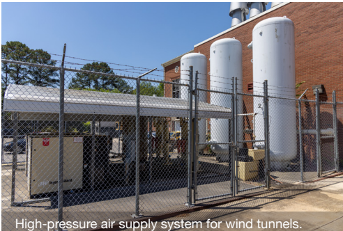
High-pressure air supply system for wind tunnels.
